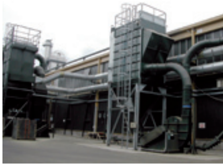
Filter chamber performance monitored via a networked Electrodynamic System
